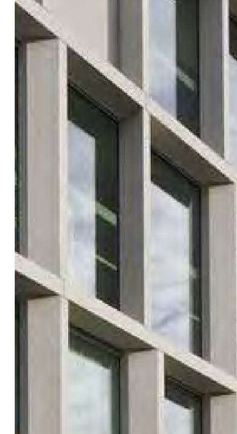
CONCRETE TYPE 2 Precast concrete frame. Colour white equal to Dulux 'Hog Bristle Quarter'.
